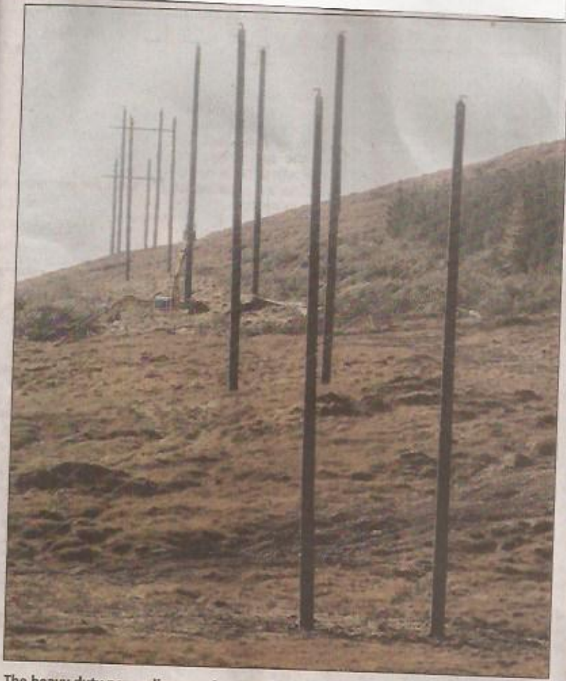
The heavy duty power lines on the site of the proposed windfarm on the outskirts of Glenties. Photo Brian McDaid. 1510bd110
